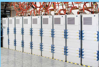
The most compact transmitter of its type, but still enormous. Nine racks are needed to provide the required output power, including standby capacity.
